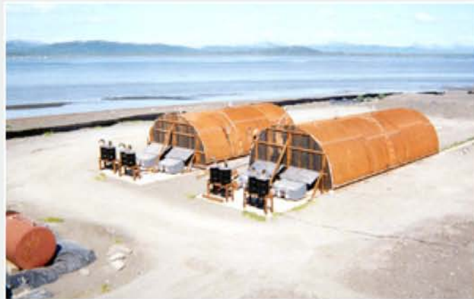
The Evaporative Desorption systems are in operation on-site at Togiak Bay, Alaska.
