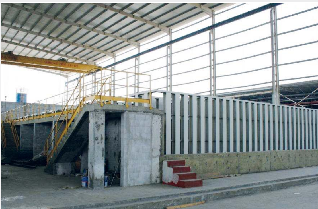
A hall was built specially for the huge galvanisation plant.
