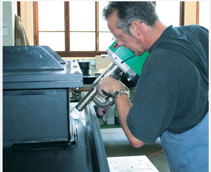
Extrusion joining the inspection hatch on to the bowed PE wall element using a WELDPLAST S.4 .
