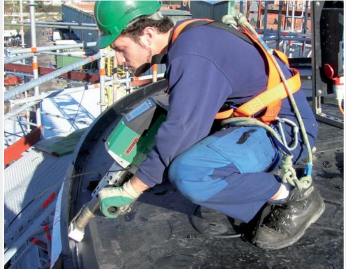
Connecting the wall and roof elements in Spain with a WELDPLAST EC 4.
