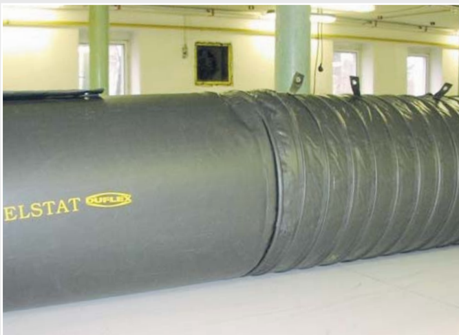
Connecting high-pressure and low-pressure air ducts.
