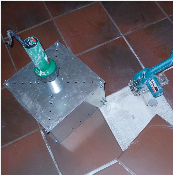
Non-destructive removal of floor and wall tiles with SysTeSan and the ELECTRON hot air blower from Leister.
