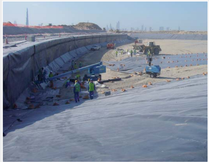
A small section of the enormous installation. On the left in the background is the «Burj Dubai».
