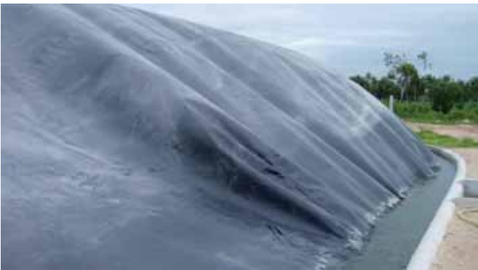
Gas extraction plant in Austria
